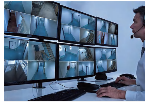
Surveillance Room & Monitoring Room
